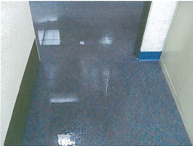
The Flood of January 2008
