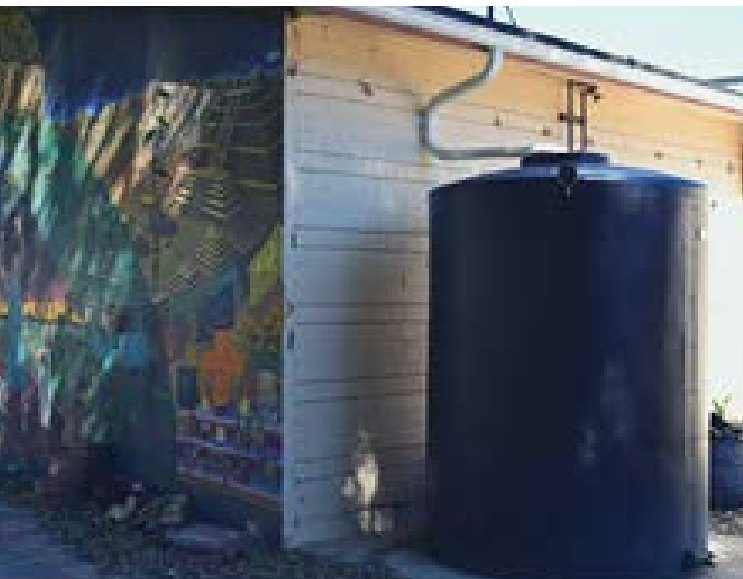
Low Impact Development (LID) Design Features Water Cistern at Cal State-Northridge
